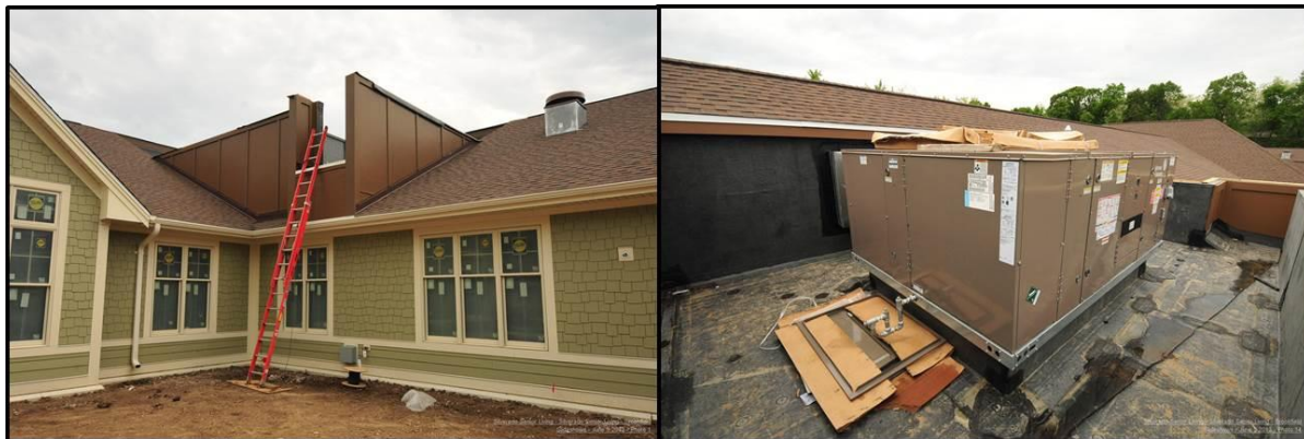
Figure 9 – Rooftop Mechanical Area (left) and RTU for Quadrant D (right)
